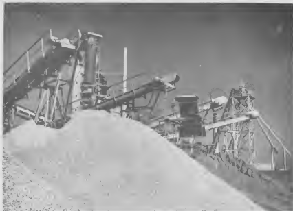
ROCK AND sand pile up on the seaward side of the Concrete Plant. The conveyors drop fresh stocks on the pile as needed, and just incidentally form interesting patterns against the sky for the photographer.
